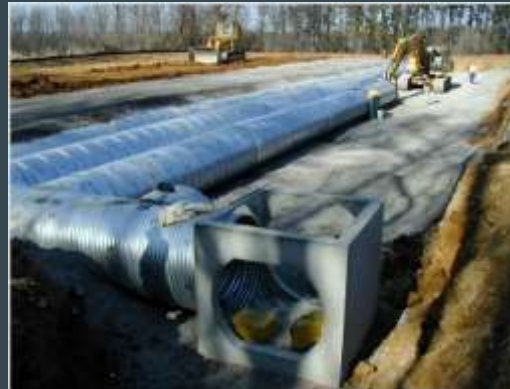
1 of 32 Subsurface Detention Ponds to reduce peak runoff rates and filter trash
